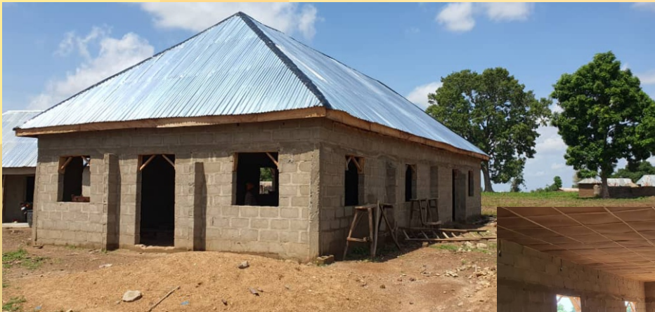
Kebbi State. Angwan Dorowa Mission church building project and Pastor's house under construction.
