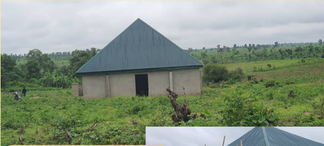
Nasarawa State. Kwanta Mission Church building project with, borehole and Pastor's house under construction.
