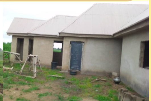
Nasarawa State. Angwan Shaho Mission Church building project with, borehole and Pastor's house under construction.
